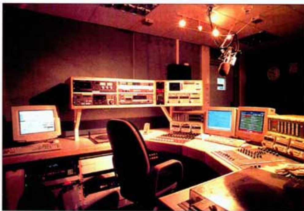
All the studios at Egton House are based around Eela consoles and SADiEs
